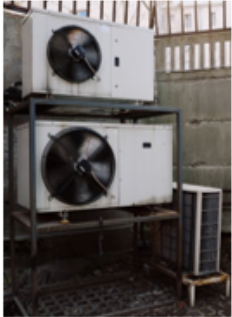
(Figure 2: Old/outdated HVAC equipment to be replaced)
